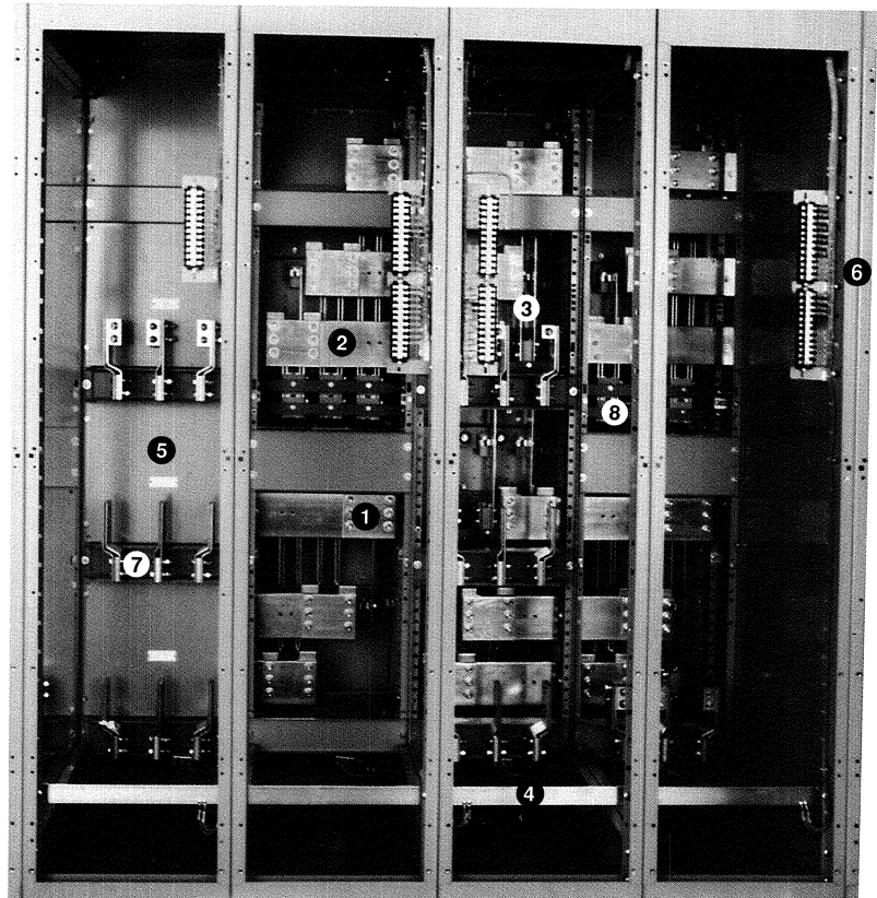
Rear view of a completed DS switchgear assembly
